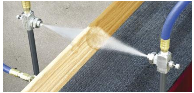
(2) Model ER1020SS atomizing nozzles are used to apply a fire retardant coating to wood trim.
